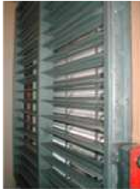
Motorized registers for air in/out/mix
